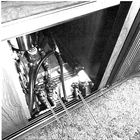
Water Drain Valves Galley
